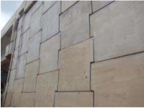
(a) Bulging/leaning of RS wall fascia
