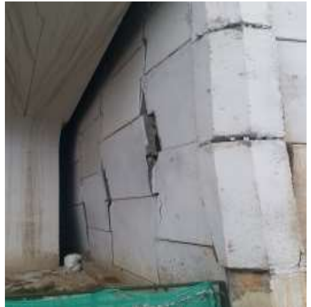
(h) Severe bulging/leaning of abutment fascia and severe dislocation of Abutment face panels
