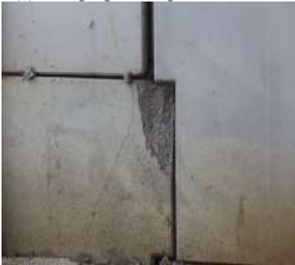
(c) Cracking of Abutment fascia panels
