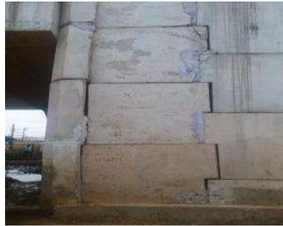
(b) Dislocation of Edge and RS wall panels
