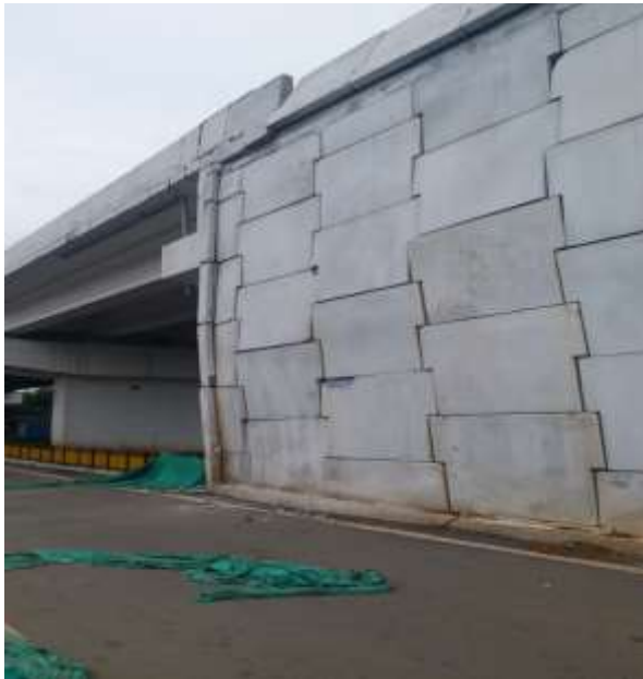
(g) Dislocation of RS wall panels
