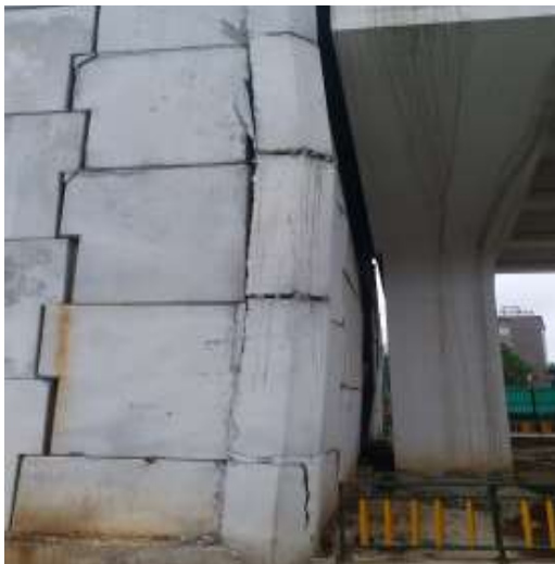
(e) Severe dislocation of edge panels and Bulging of abutment
