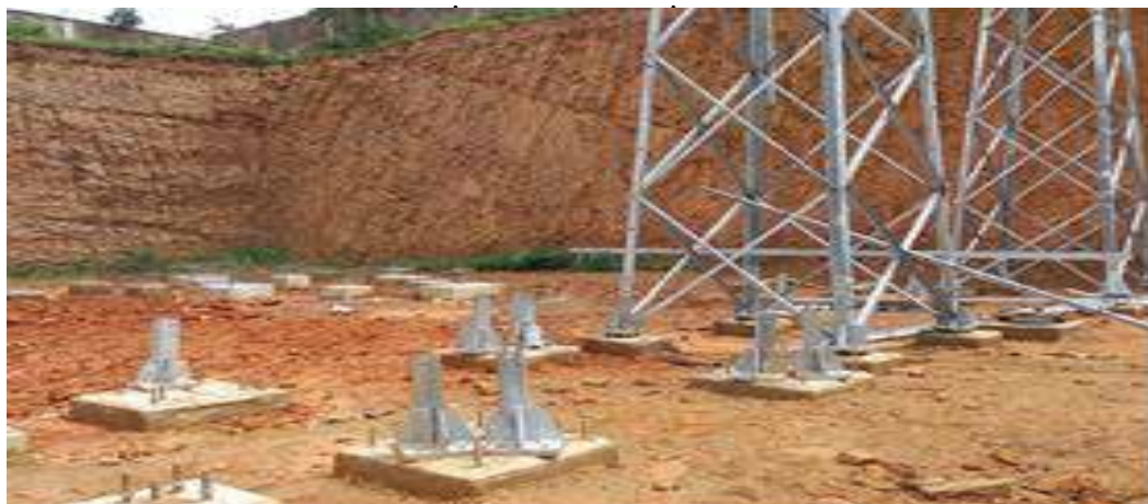
Fig. 4 : Proximity of substation to vertical cliff
