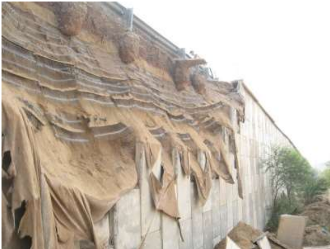
Fig. 2 : Structure showing no reinforcement at top panel
